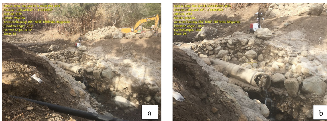
Fig. 4. (a) Upstream view of San Ysidro creek debris-catch basin culvert, showing damage sustained during the January 9, 2018 debris flow event. (b) Detail view of damage to culvert.
