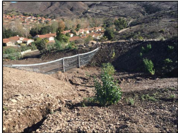
Fig 4. UX net with posts for wider channels Camarillo, California.
