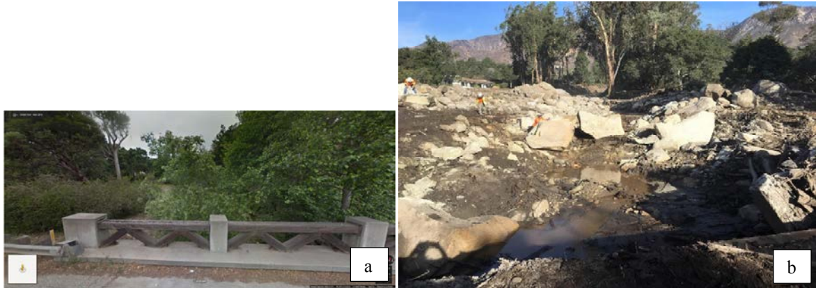
Fig. 10. (a) Looking upstream from SR 192 bridge at San Ysidro Creek, pre-event. Google Maps Street View image taken May 2016 (© Google). (b) Post-event photo taken from same location as Fig. 10a on January 18, 2018. Note a significant amount of debris had already been removed from stream channel.
