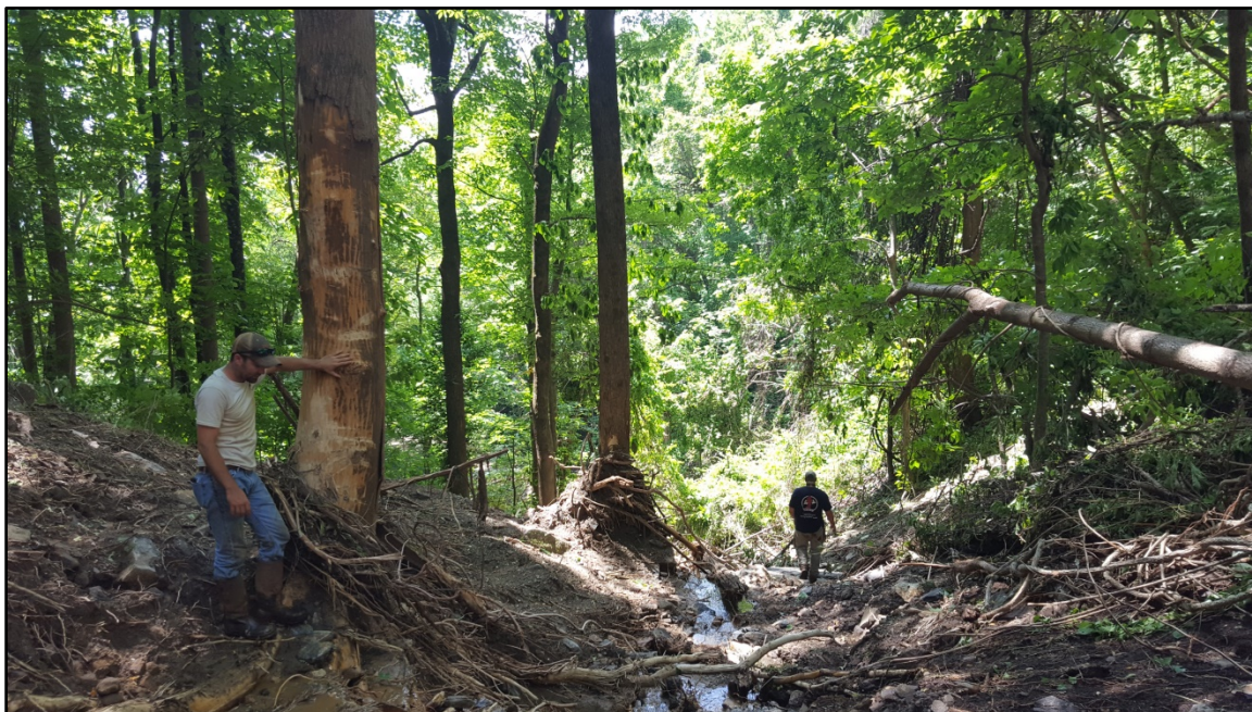
Fig. 4. Downstream view of debris flow in the Meadowlark Drive area. Tree nick marks can be observed twice as high as the height of the worker by the tree, approximately 3.6 meters high (12 feet).
