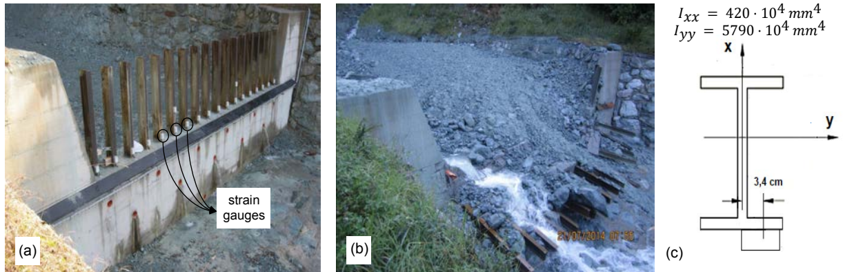
Fig 1. Illustration of the sectional dam used as study case, respectively before (a) and after (b) the collapse happened on 20/07/2014; (c) the cross section of the steel beams. The pictures are courtesy of Regione Autonoma Valle d'Aosta.
