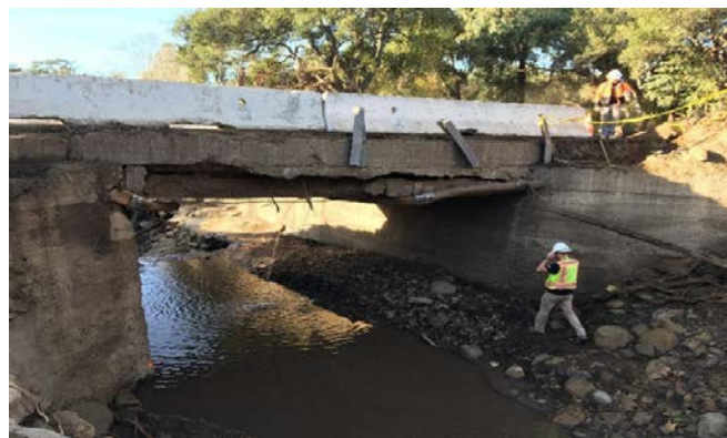
Fig. 6. Montecito Creek Bridge at SR 192, January 18, 2018. Note lack of scour behind/below abutment wingwalls. Significant amounts of debris had been removed from the channel at the time of this photo.
