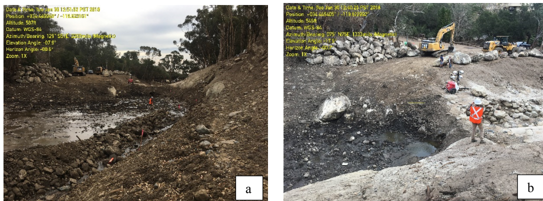
Fig. 3. (a) View downstream showing remaining sediment, boulders, and woody debris within San Ysidro creek debris basin during clean out operations. (b) Cross stream view of debris basin outlet and stock pile of boulders removed from San Ysidro creek debris basin during clean out operations.
