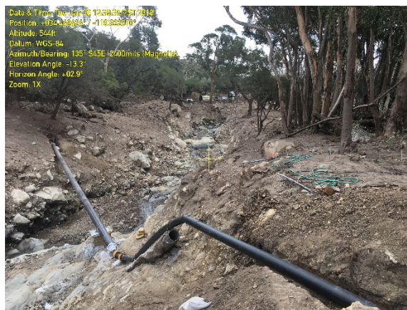
Fig. 12. Downstream view of temporary repair of the “Highline” water main by Montecito Water District. Sections of the previously buried water main were exposed due to channel scour during the debris flow event within San Ysidro Creek.
