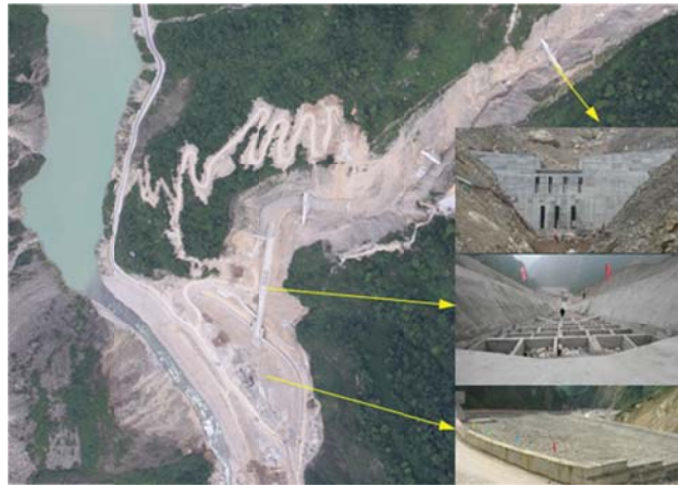
Fig. 8 Application of the debris-flow mitigation structures in Xiaogangjian gully, Sichuan Province, China
