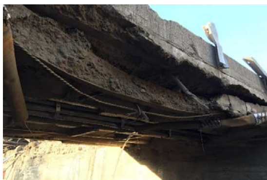
Fig. 8. Damaged girder and utilities, upstream side of Montecito Creek bridge at SR 192. Note exposed girder reinforcement consists of embedded steel beam section and continuously twisted steel bar; steel beam sections exhibit residual curvature.
