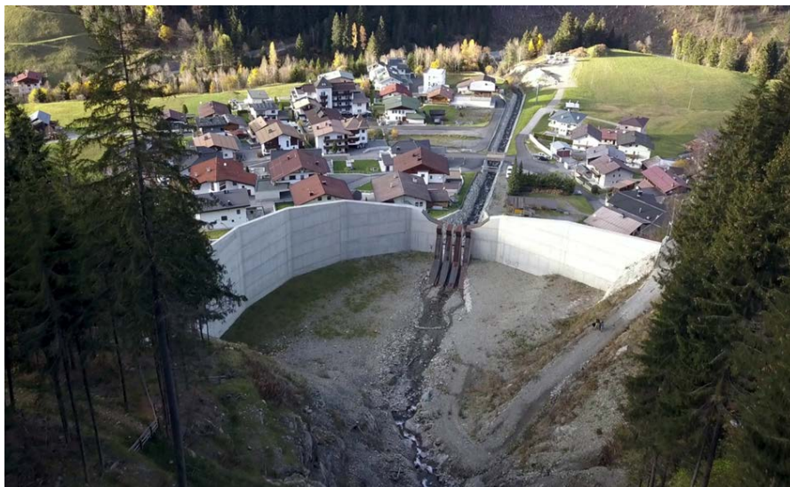
Fig. 7. Recently completed debris-flow barrier with the sediment retention basin (Schallerbach, Tyrol), designed according to the ONR National Guidelines.
