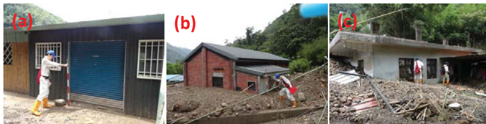
Fig. 3. Damaged building and damage class applying Jakob et al. (2012) method: (a) #4, metal sheet structure with damage class I; (b) #11, brick structure with damage class II; (c) #13, reinforced concrete structure with damage class III (photo: Hsu, C.H.)
