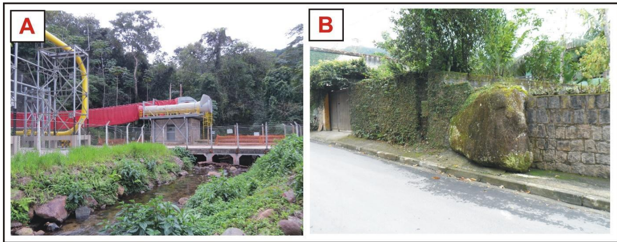
Fig. 6. (a) The Gas Treatment Unit (UTGCA), from PETROBRAS installed in Pau d'algo watershed, with precautionary measures to debris-flows damage, as the elevation of the pipes (left) and culverts to withstand debris-flow passage (right); (b) boulder used as part of the construction of a wall from a house, in Guaxinduba watershed.
