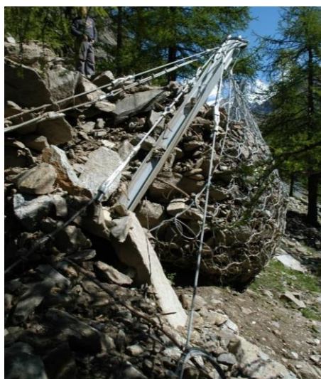
Fig. 2. Barrier clogged by rocks installed in the Alps (Courtesy of Maccaferri)
