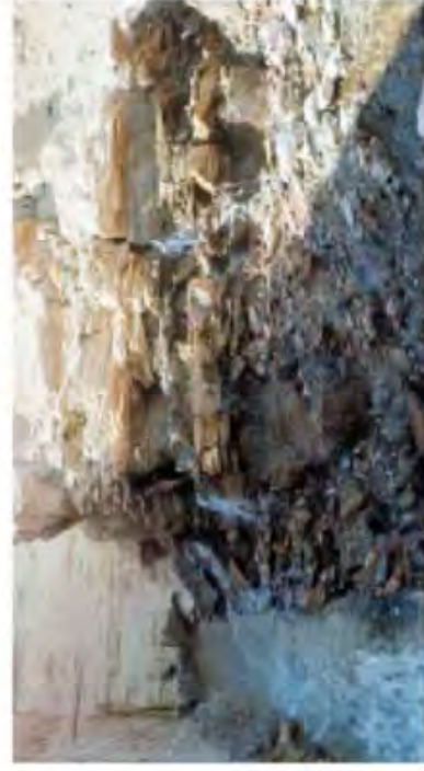
Fontenelle Dam Incident, Wyoming, USA from USBR
